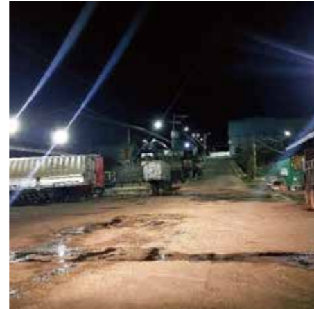
Construction site used PENEL Solar lights with 8m height in 2024 in the Philippines
