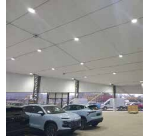
PENEL 150W LED High Bay lights were illuminating a car showroom in 2023 in Chile
