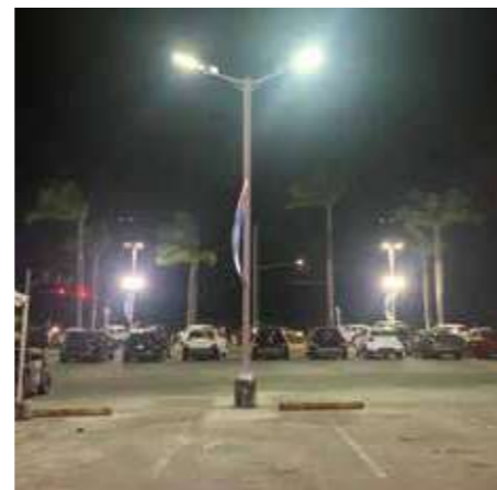
A large mall parking lot used PENEL integrated Solar streetlights with 30 feet pole in 2022 in USA
