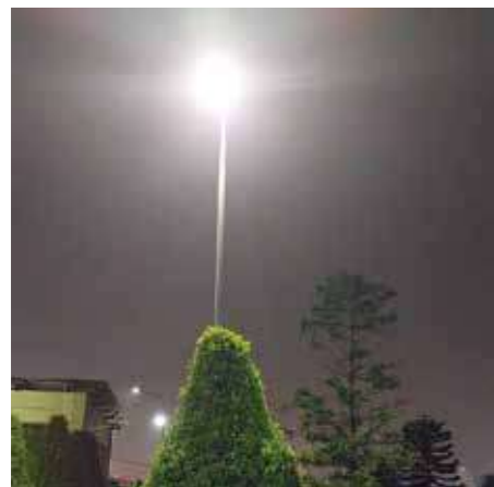
PENEL Integrated Solar Streetlights were lighting up at night in 2022 in Indonesia
