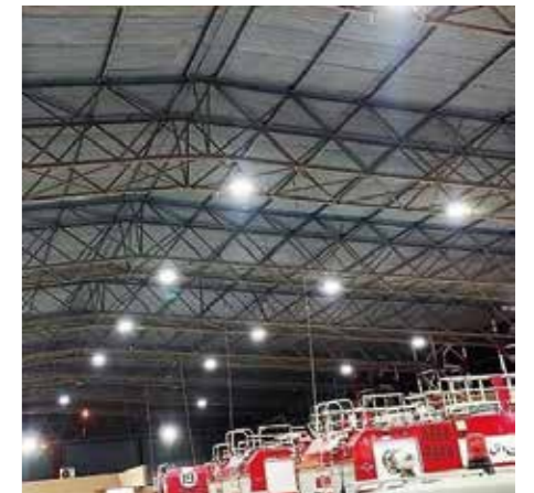
PENEL 150W LED High Bay lights were illuminating the fire protection district of Civil aviation administration in 2022 in Pakistan
