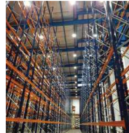
PENEL 150W LED High Bay lights were illuminating a warehouse at 14m height in 2023 in Indonesia
