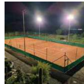
New tennis court used PENEL 250W LED Sports lights in 2024 in Italy
