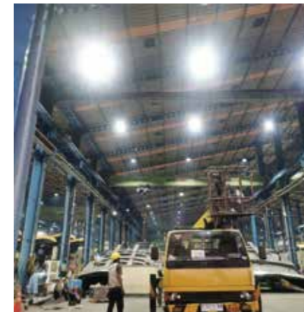
PENEL 150W LED High Bay lights were illuminating a workshop in 2023 in Indonesia
