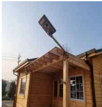
PENEL Integrated Solar streetlights were installed in 2023 in Korea
