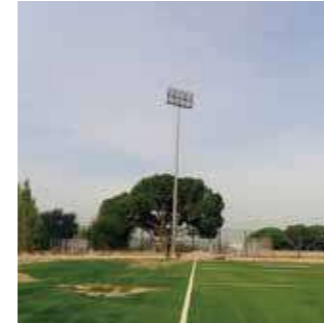
Football field used PENEL 1500W sports lights in 2025 in Lebanon
