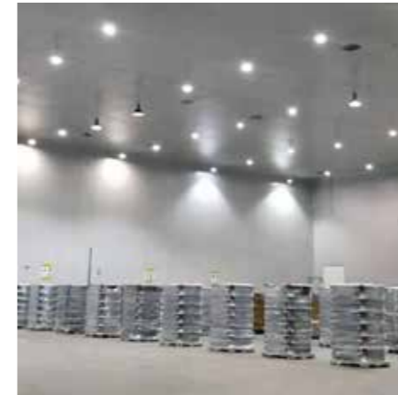
PENEL 200W/100W LED High Bay lights were illuminating a Quilmes beer warehouse in 2024 in Argentina.
